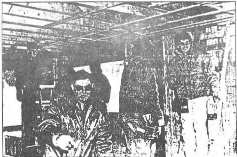
TEAMWORK — Silver Lake Regional High School students and their instructors work inside the house they are building in Halifax. (Staff photo by Sara Altherr)
